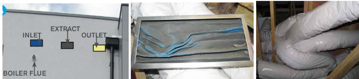
Figure 2a), close location of inlet, outlet and boiler flue; 2b) dirty filter; 2c) constricted flexible duct
